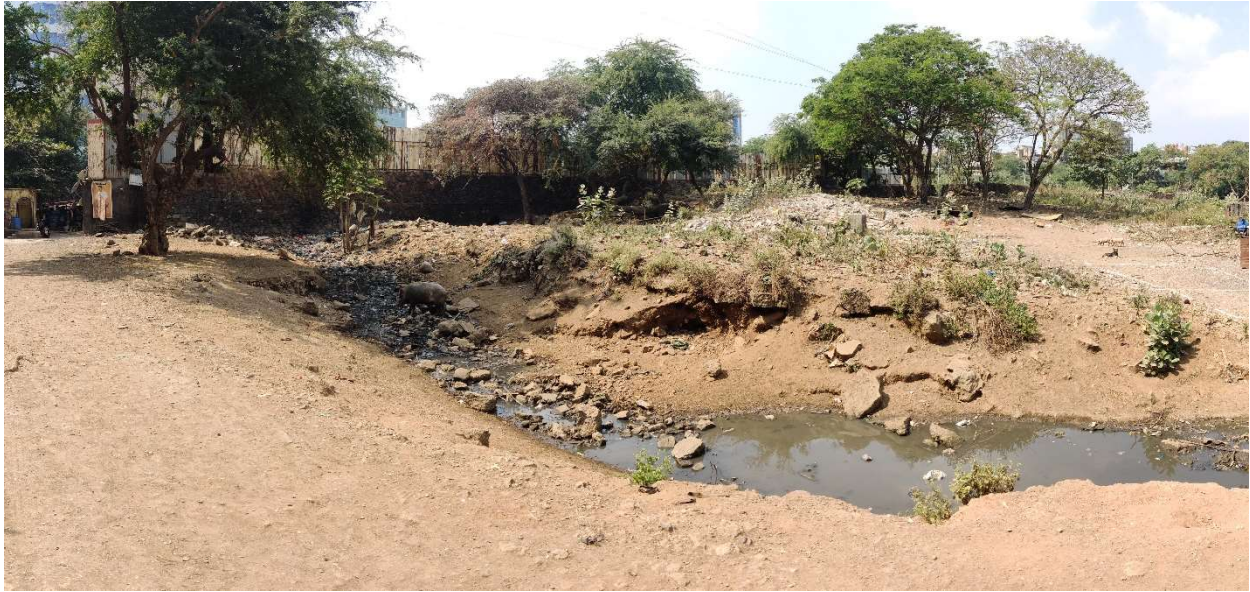
Figure 13: Storm water outfall
