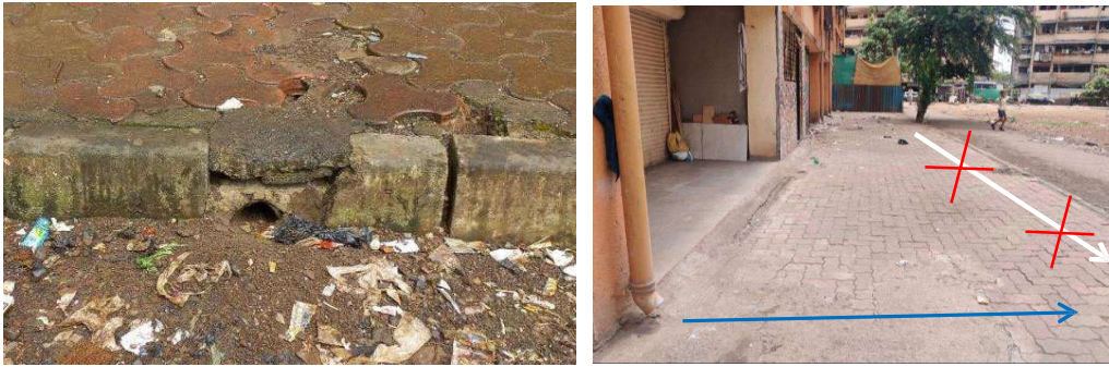
Figure 3.12 Block drain pipes under pathways around the maidan. (Right) Crossed lines indicate previously functional drainagae lines closed by residents. Blue is the flow of rooftop rainwater
